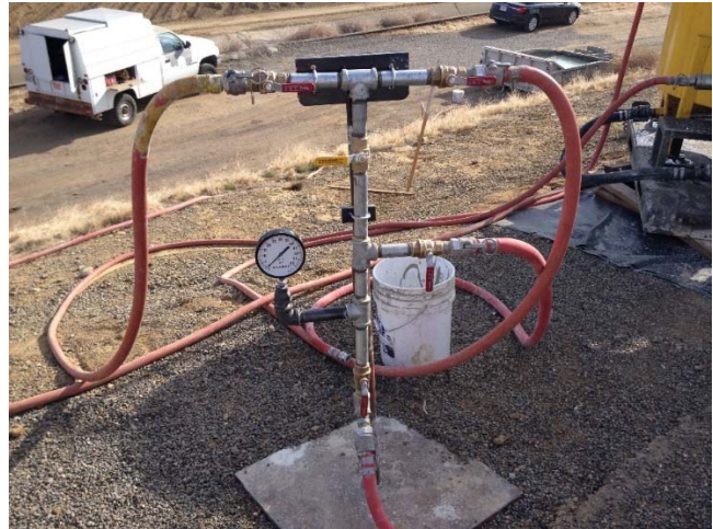
Figure 18. Example of a grout manifold to allow for grout recirculation and control of flow and pressures to the grout hole.
