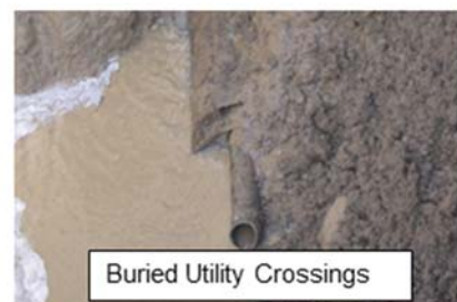
Figure 2. Examples of embankment issues.
