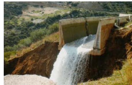
Figure 22. Examples of slope instability.
