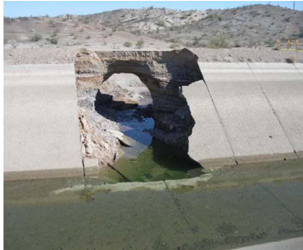
Figure 1. Example of a recent canal failure.
