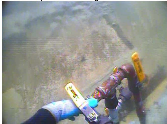
Figure 20. Diver grouting voids beneath the liner. Note grout “bleeding” from vent hole further up the liner slope.
