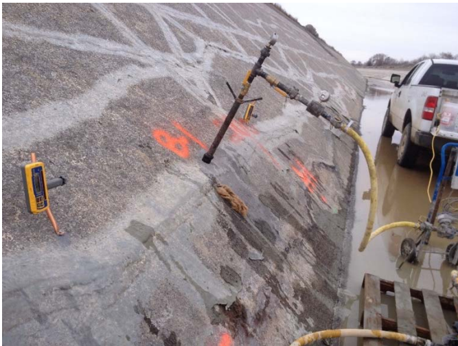
Figure 19. Example of grouting beneath concrete lining to fill voids and seepage paths. Note laser levels used to monitor liner uplift.
