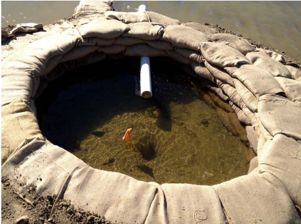
Figure 9. Example of a ring dike constructed around a sand boil to reduce the exit gradient and measure the seepage flow.
