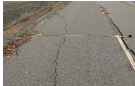
Figure 26. Examples of signs of slope instability.
