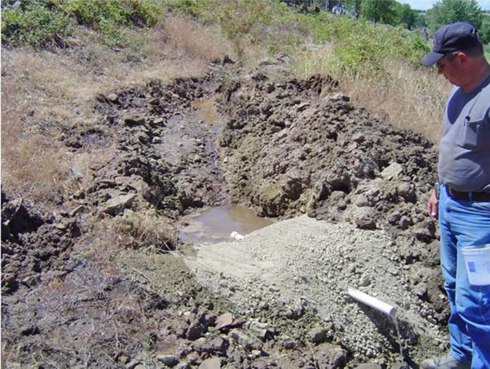
Figure 8. Example of initial measures used to collect and measure seepage flows.
