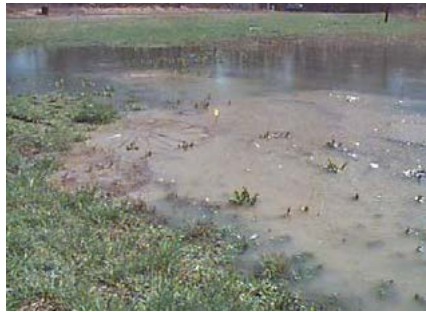
Figure 7. Seepage indicating possible burrows.
