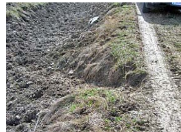
Figure 5. Livestock damage to canal embankment.
